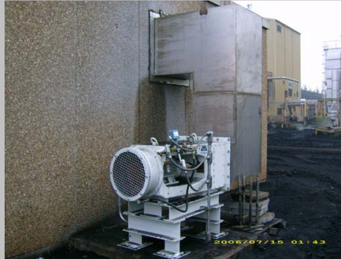
Ambient coal yard air is pulled into the Engart Extractor by its integrated impeller, cleaned, and then exhausted into the MCC Room.
