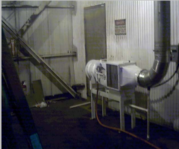
Ambient plant air is pulled into the Engart Extractor by its integrated impeller, cleaned, and then exhausted into the MCC Room.
